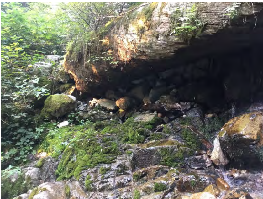
Log retaining fill not anchored on right bank
